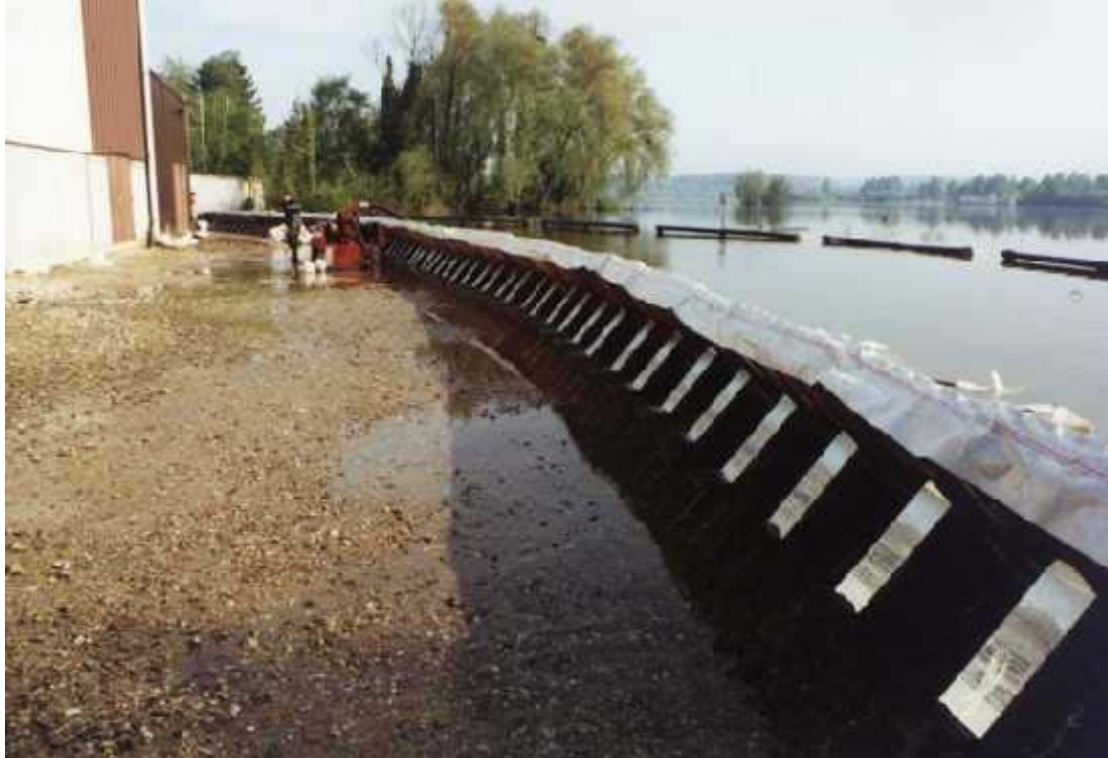
Temporary defence structure. Source: www.environment-agency.gov.uk
